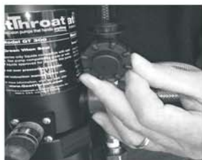
1. Open vent on pump
